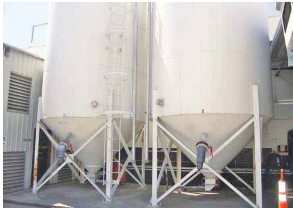
Silos where plastic pellets are stored until formed into case.
